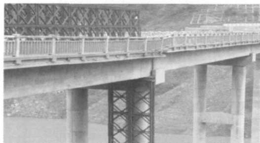
(a) 边跨接近落梁
