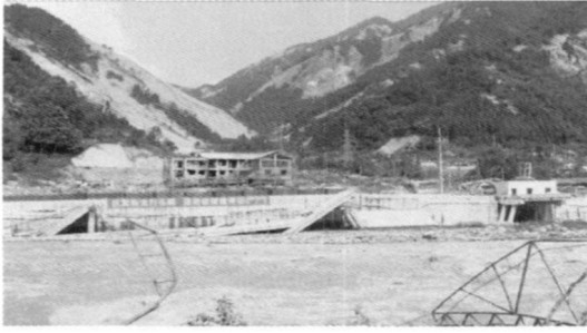
(a) 落梁倒塌
