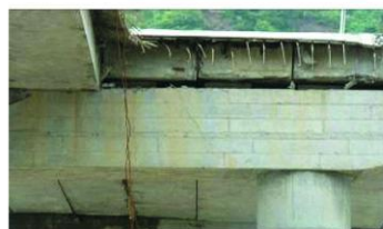
(i) 盖梁的剪切裂缝
