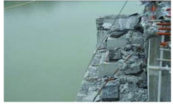
(c) 落梁处支座、挡块破坏情况
