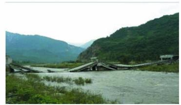
(c) 南侧2跨整体坍塌
