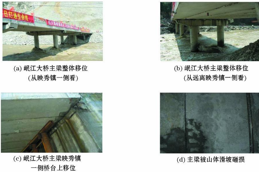
图 9 岷江大桥震害 Fig 9 Damage to Minjiang Bridge
